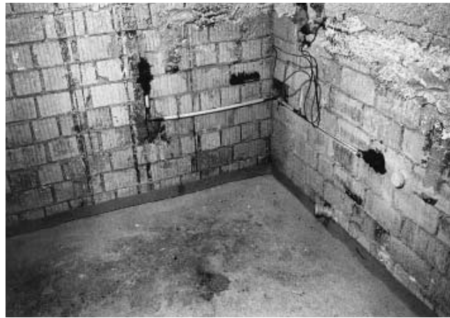
Fig. 6 Strips of insulation laid against the walls of a room to be tiled
