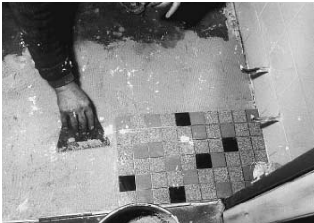
Fig. 11 Laying the ceramic tiles in a bed of mortar of 1 mm thickness
